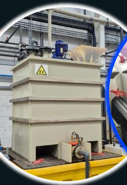
Magnet Digestion tank being operated
